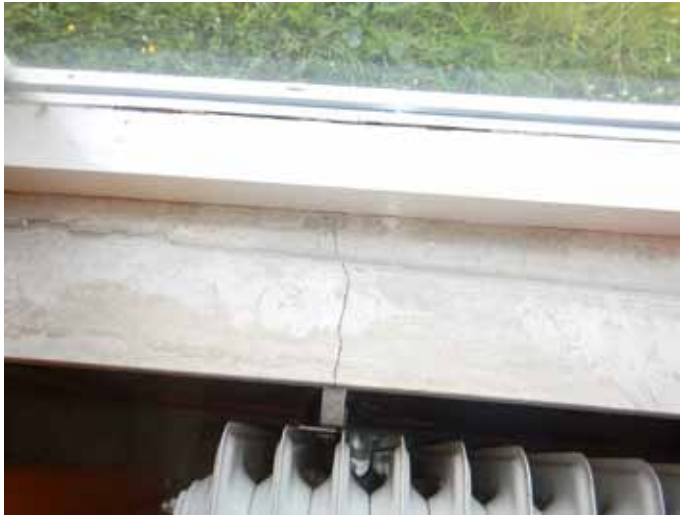
idem; gebroken vensterbank
